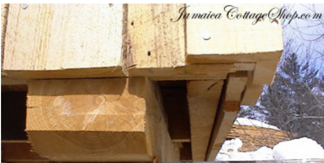
Bottom of building showing 4x6 skid placement and bottom of siding and trim
